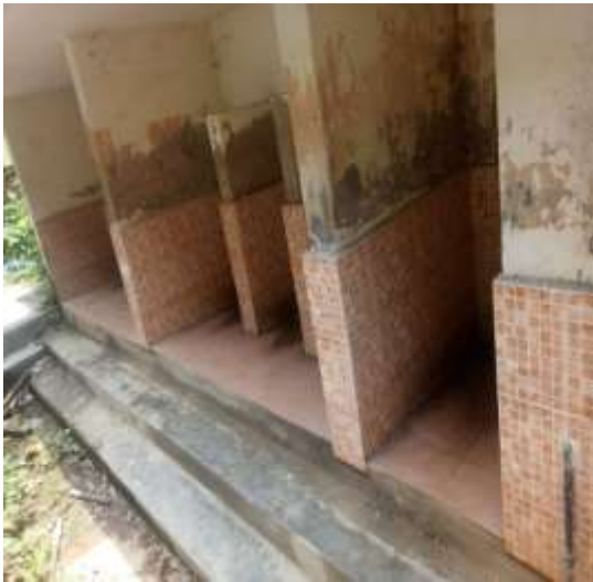
Toilet and Urinal facility
