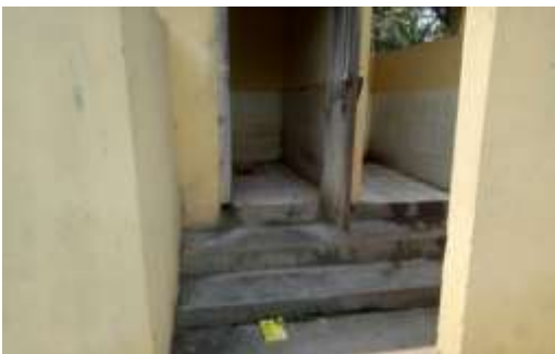
Toilet and Urinal
