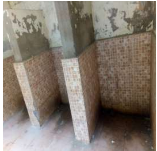
Toilet and Urinal facility
