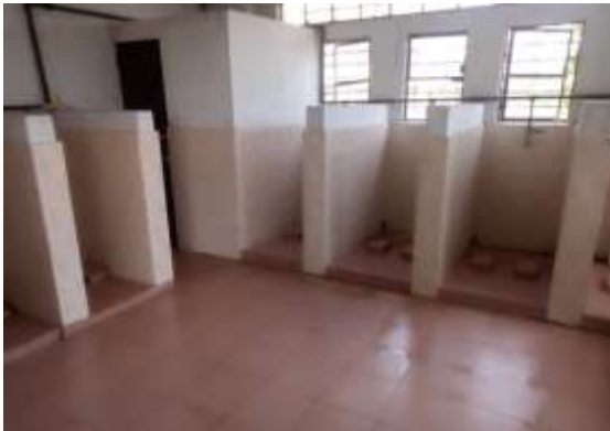
Toilet and urinal
