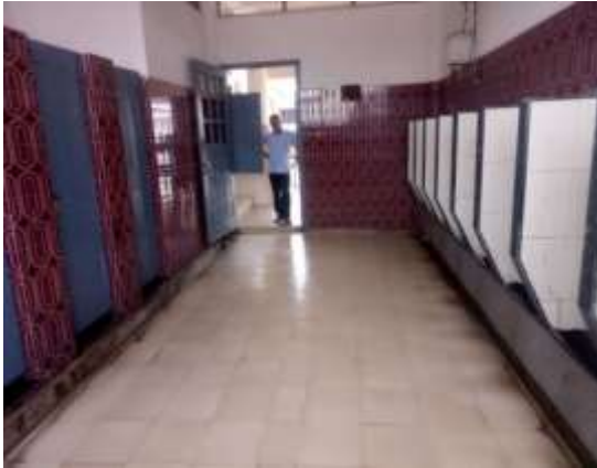
Toilet and urinal facility
