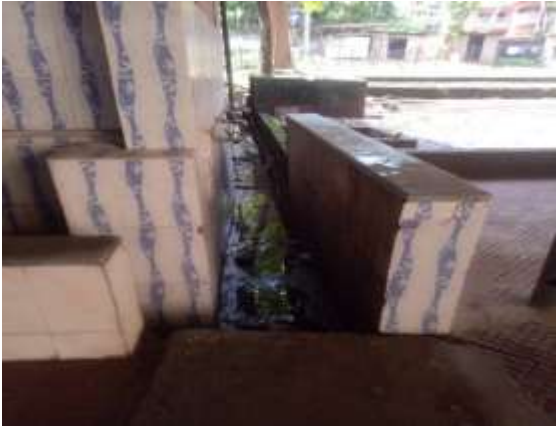
Drinking water facility
