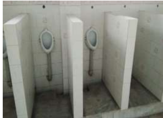
Toilet and Urinal
