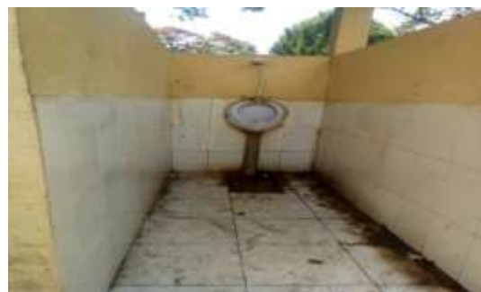
Toilet and Urinal
