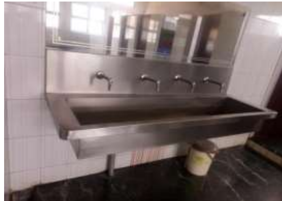
Water facility in Toilet and Urinal
