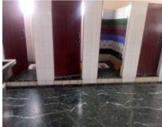
Toilet and urinal facility
