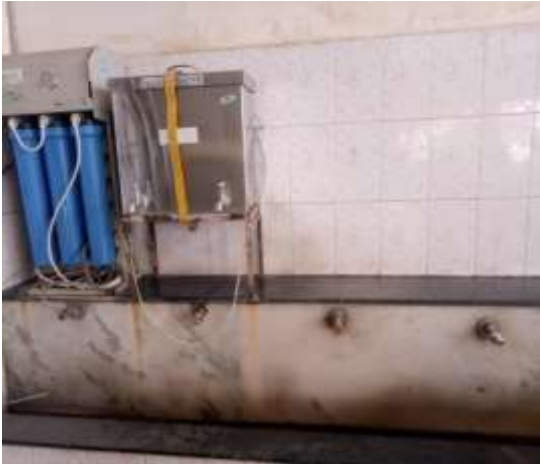
Drinking water facility
